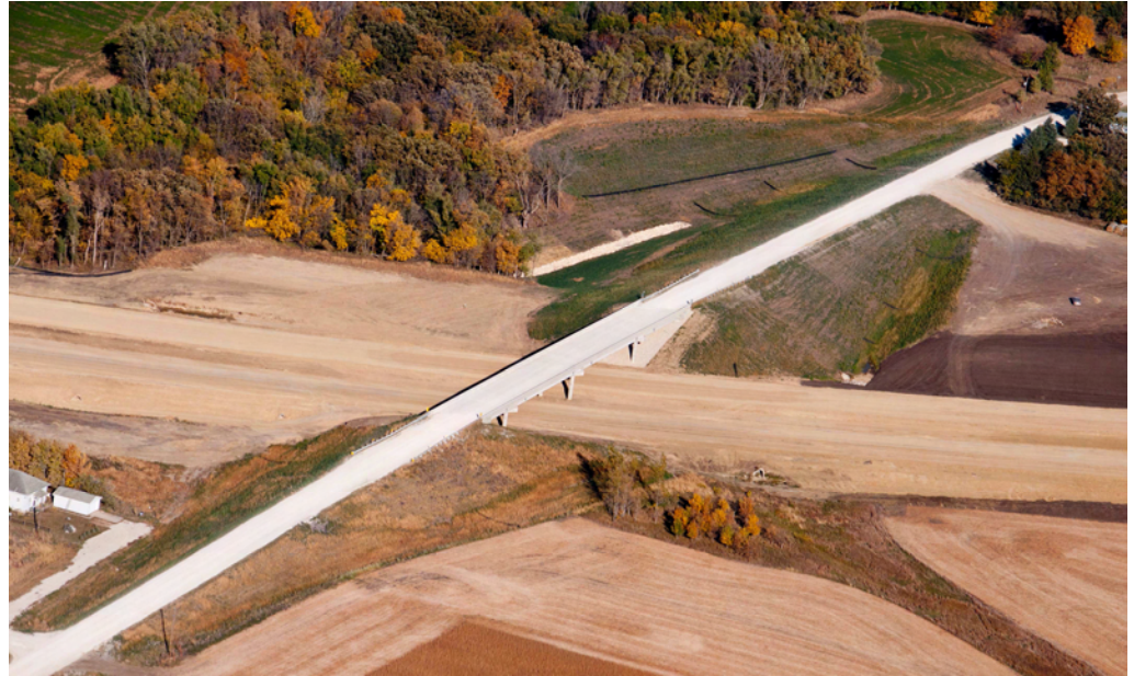
230th Street overpass is now open. This is looking eastward with the graded four lane Hwy. 20 beneath it. Photo compliments of Matt & Cindy Wallace—10/5/11)
