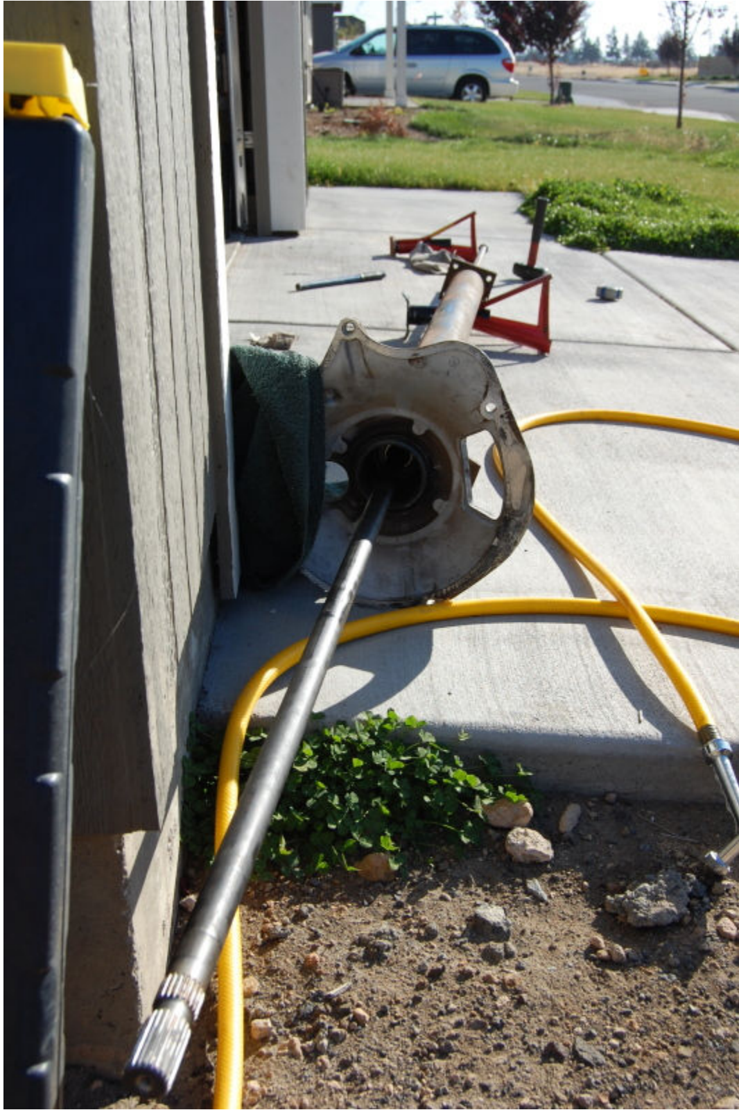
Now with the shaft out the next thing is to get the bearings out.
