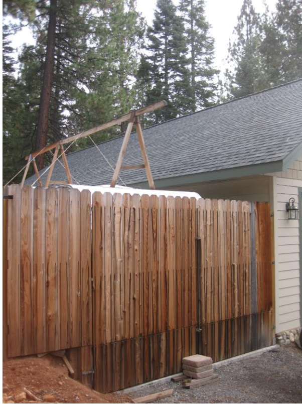
Photo 7-Wooden fence connected to a structure.
