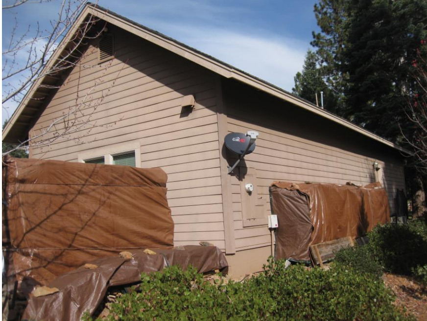
Photo 6-Firewood being stored against a structure
